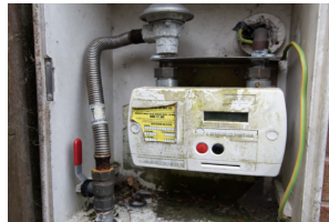
External gas meter with emergency control valve (red) P-KIIRX0 · 2026-06-06 11:50
