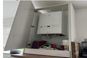
Ideal Logic combi boiler in kitchen cupboard P-XCRA83 · 2026-06-06 11:44
